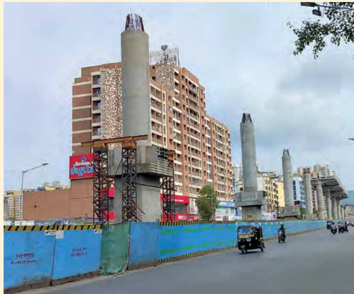
Upcoming metro projects will continue to drive demand for VT.
