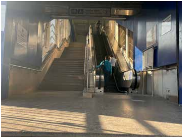
Escalators at a metro station
